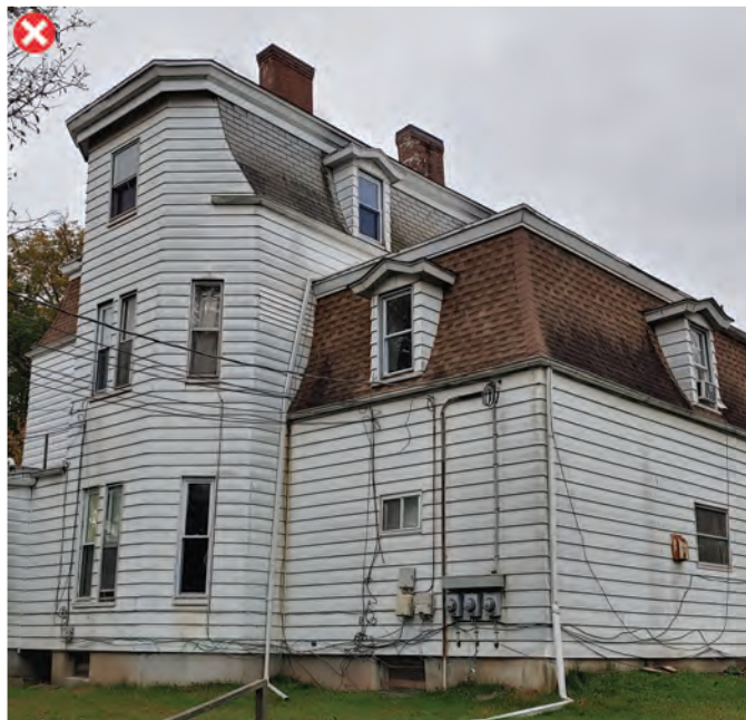
Structure is covered in vinyl siding - the impermeability of vinyl can cause condensation and degrade historic substrate
