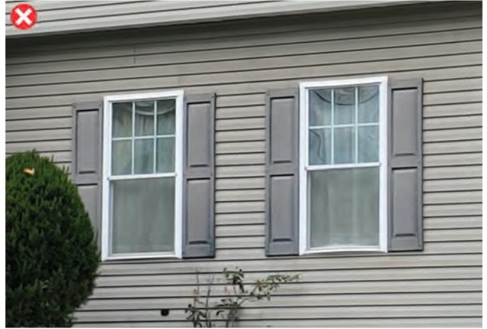
Inappropriate vinyl siding, vinyl replacement windows, and artificial decorative shutters
