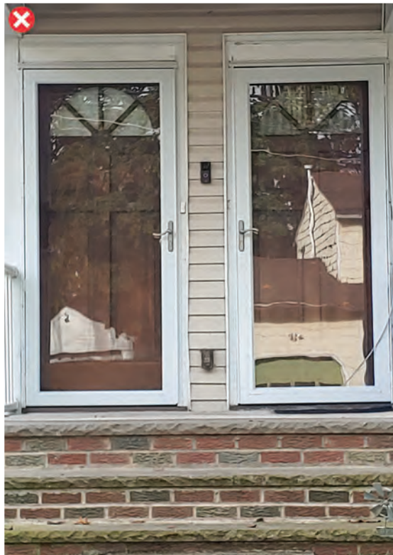
Incompatible storm door design
