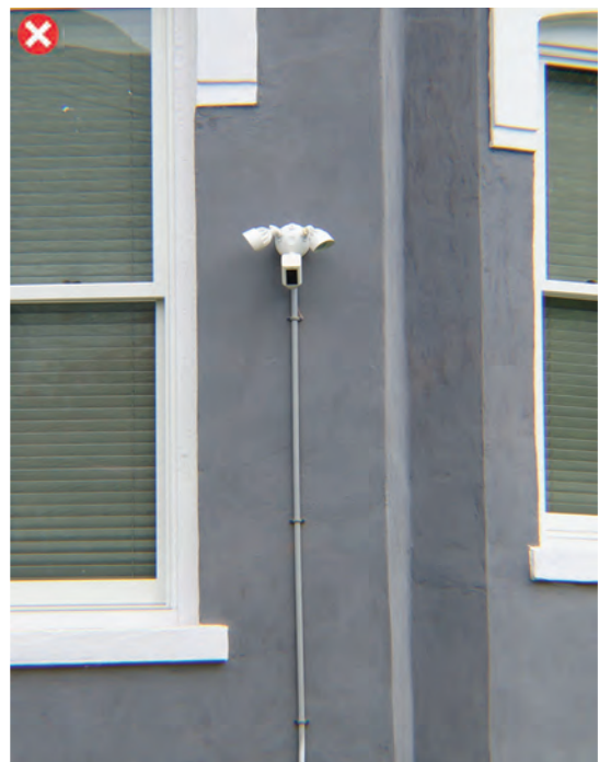
LED floodlights installed conspicuously
