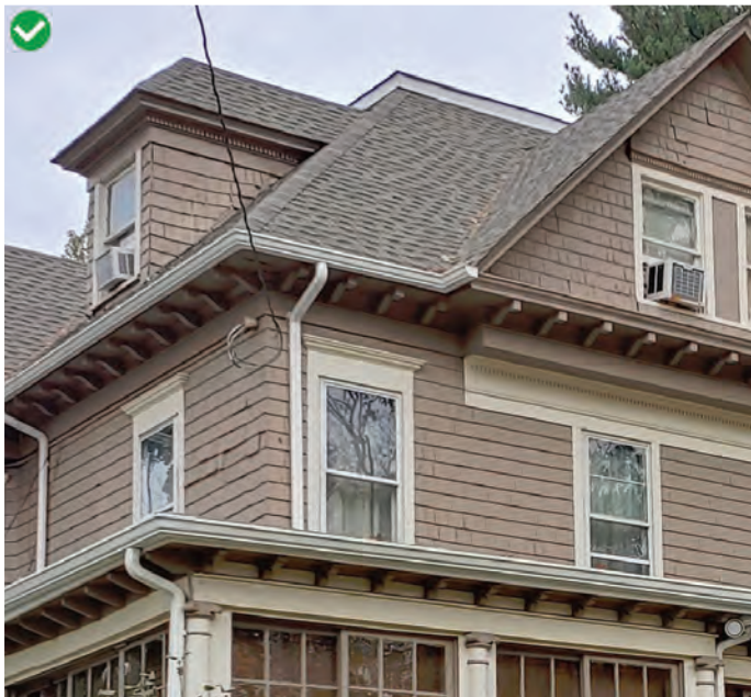
Wires attached under eaves and concealed.
