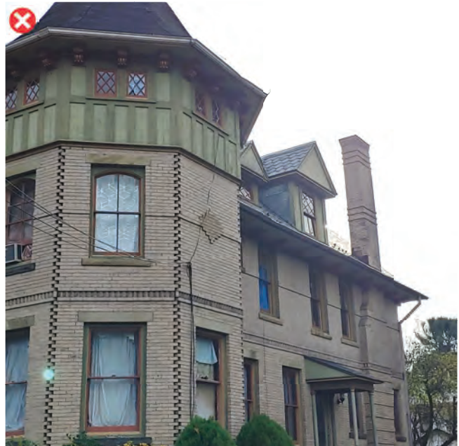
Wires attached to front elevation brickwork.
