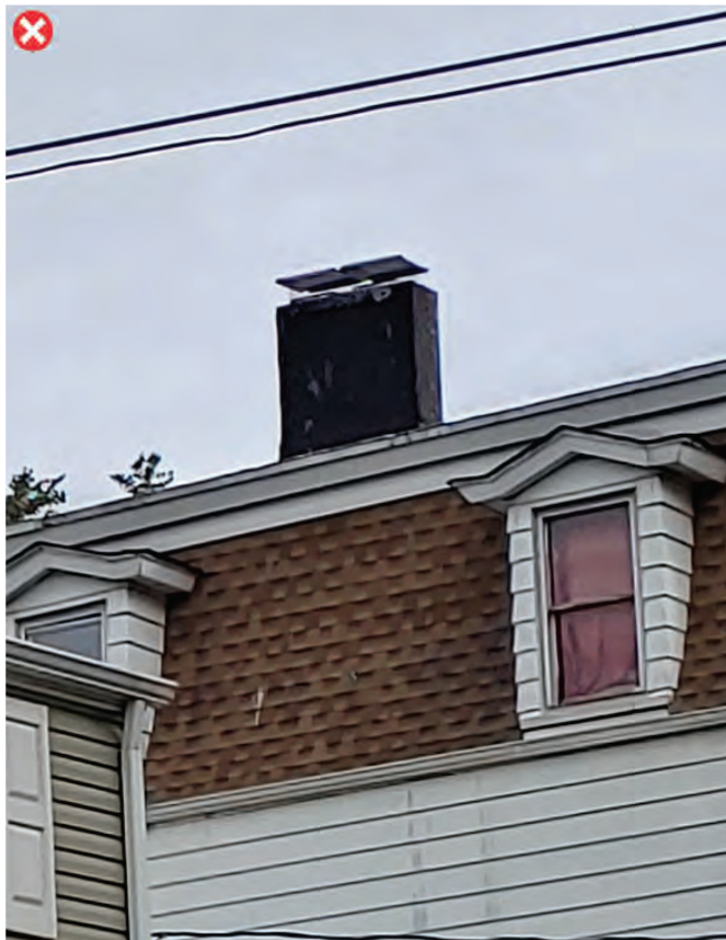
Incompatible metal chimney cap replacement; chimneys should have clay, slate, brick or stone caps
