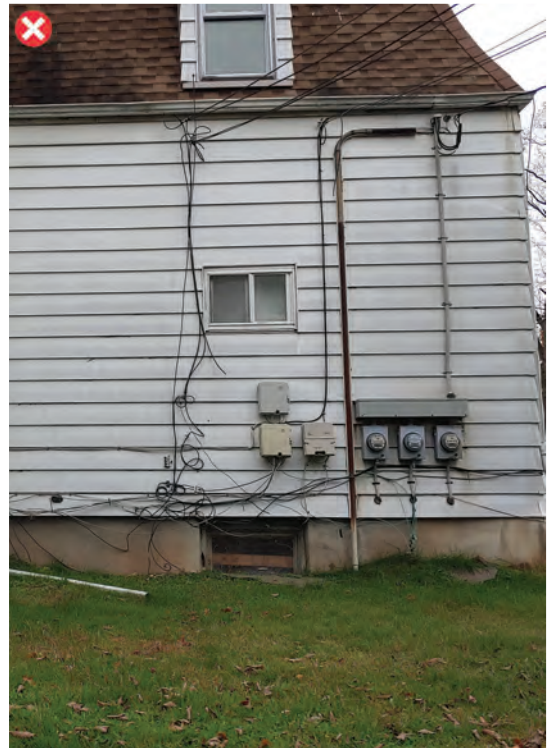
Wires not concealed
