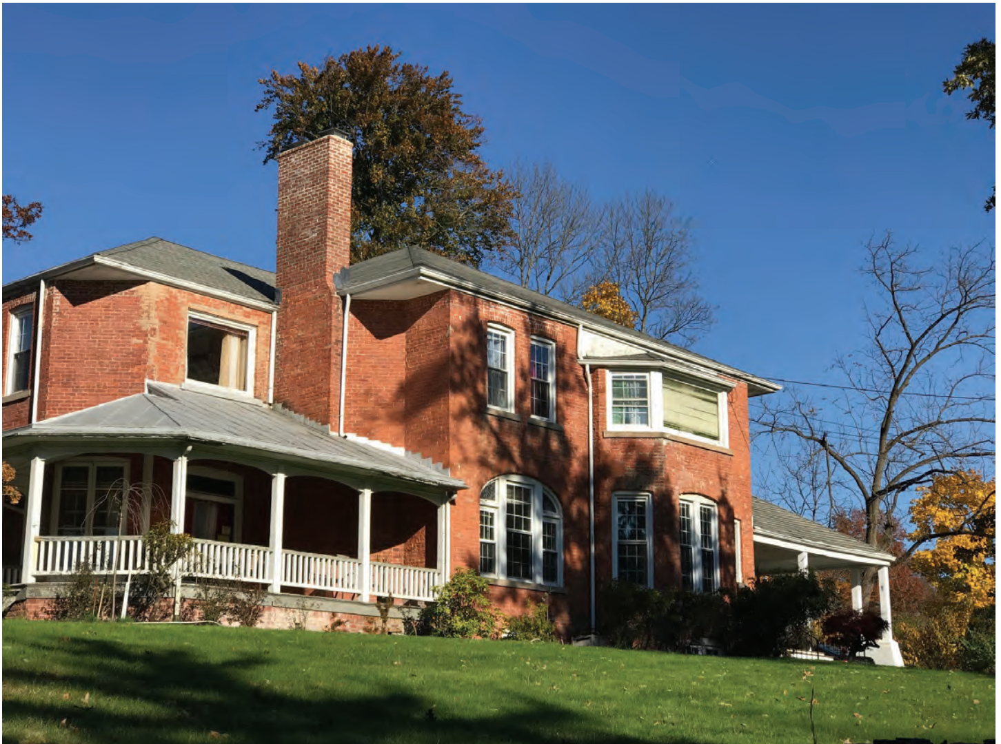
Rockview Terrace residence showing common masonry conditions on such as wearing of mortar joints and brick faces, and efflorescence (white deposits from salt in mortar)
