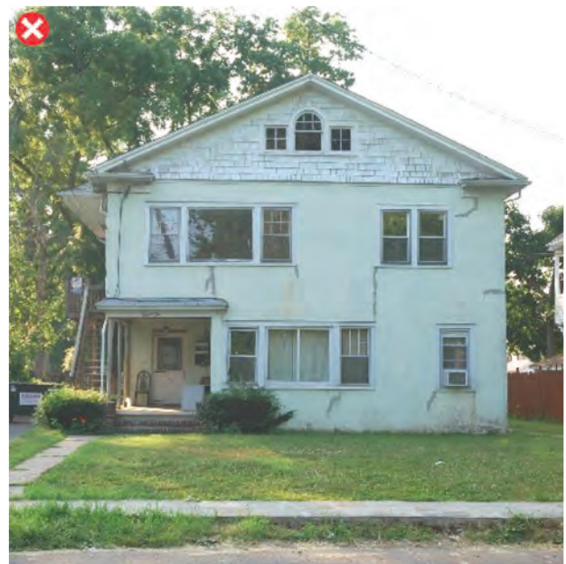
Stucco is in disrepair and has not been maintained; water and vegetation have caused discoloration
