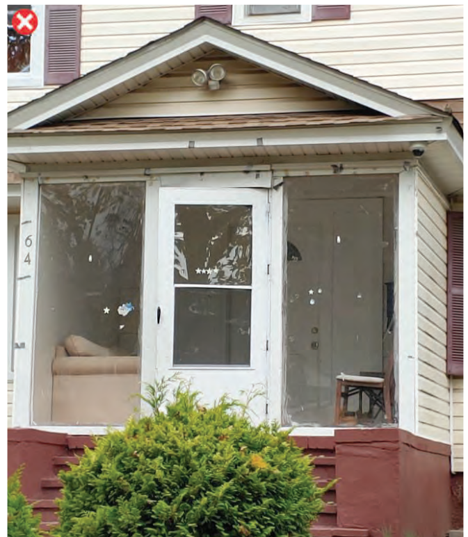
Architectural features were not preserved and porch has been filled in with incompatible material
