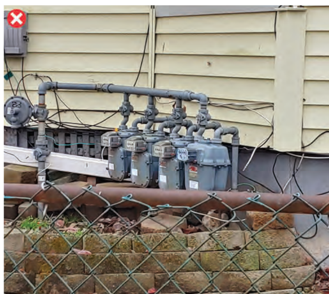
Exposed gas utility
