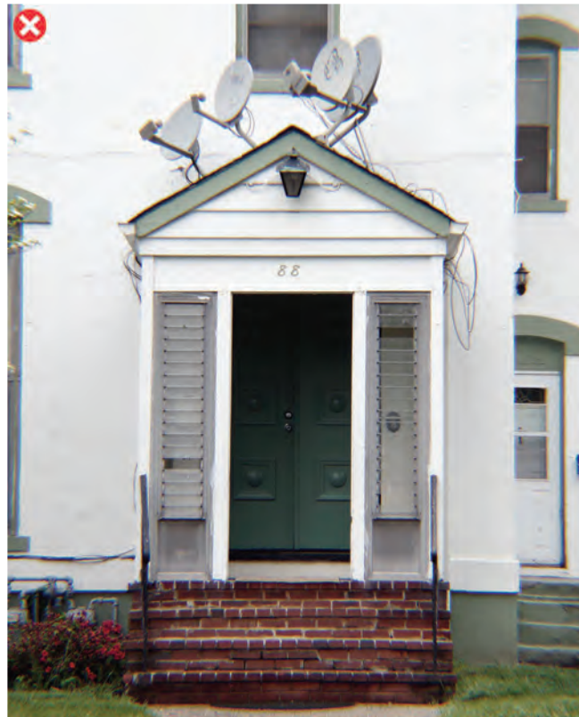
Satellite dishes installed above primary entrance
