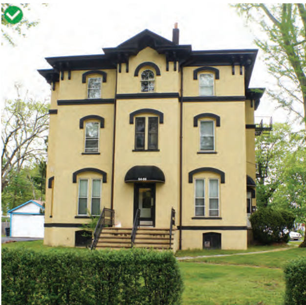
This textured stucco siding is in good repair with details appropriately highlighted
