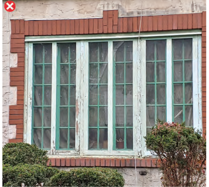
Poorly maintained wood casement windows
